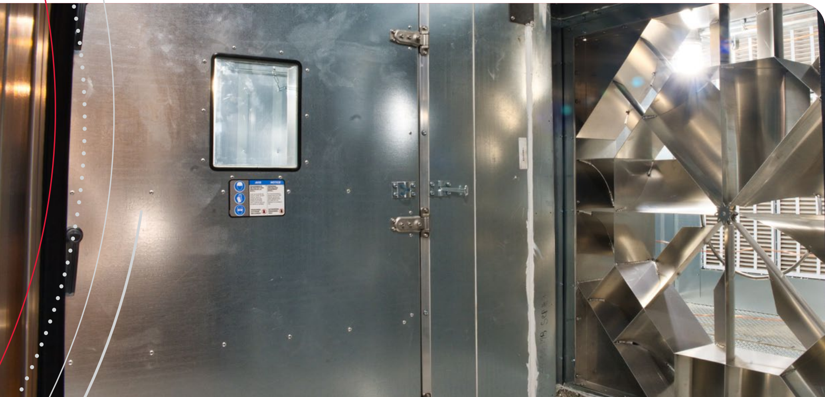
Ventrol access door located beside Blender Products air blender component.
