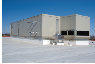
Packaged Rooftop Units
